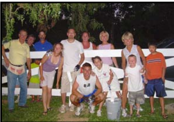
Twelve family members of Virginia Turner on Rollington Road gathered recently to build their mother a Pewee Valley fence. It took the hard-working group approximately one week to complete the fence on two sides of her two-acre property.
